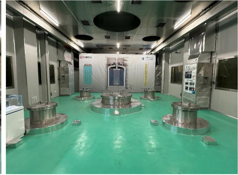
Clean room above LIN tank
